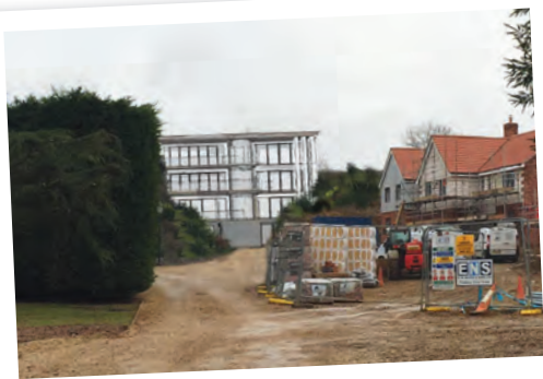
The house's location and orientation on the site has been carefully planned
